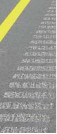
Photo of a rumble strip
